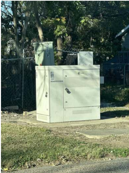
DSL Cabinet (E Williams St.)
