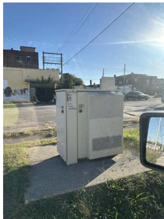
DSL Cabinet (South Danville)
